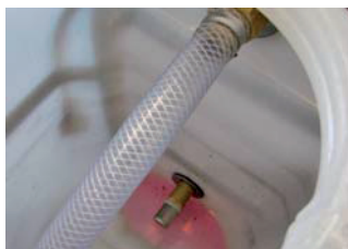
filter inside tank
